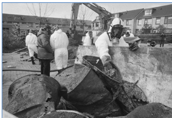
Photo 1. Chemical waste excavated in Lekkerkerk (Date: 23 April 1980)
